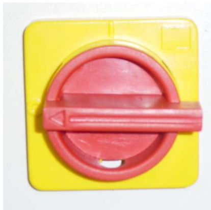
Figure 15. MAIN POWER SWITCH IN THE OFF POSITION.
