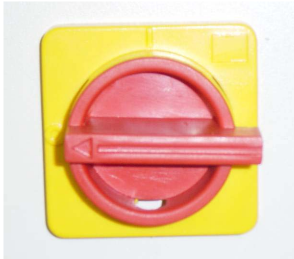
Figure 8. MAIN DISCONNECT SWITCH ON THE ELECTRICAL ENCLOSURE
