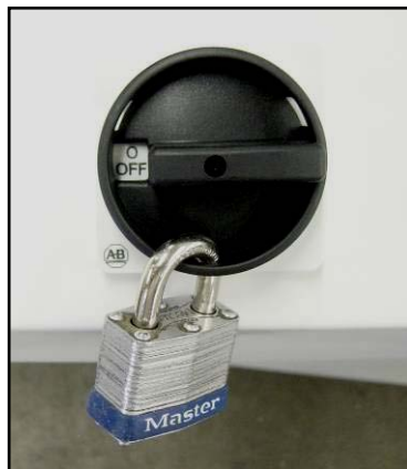
Figure 16. MAIN POWER SWITCH IN THE LOCKED POSITION.
